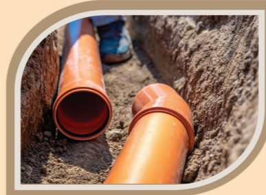
Underground Drainage System
